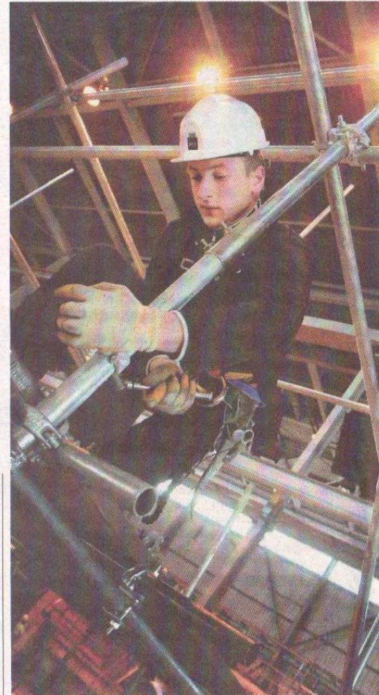
>> UP THERE LIKE A MONKEY A Simian Risk Management trainee at work in the company's new warehouse centre
